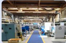
Air Flow Monitoring
