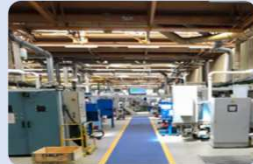
Air Flow Monitoring
